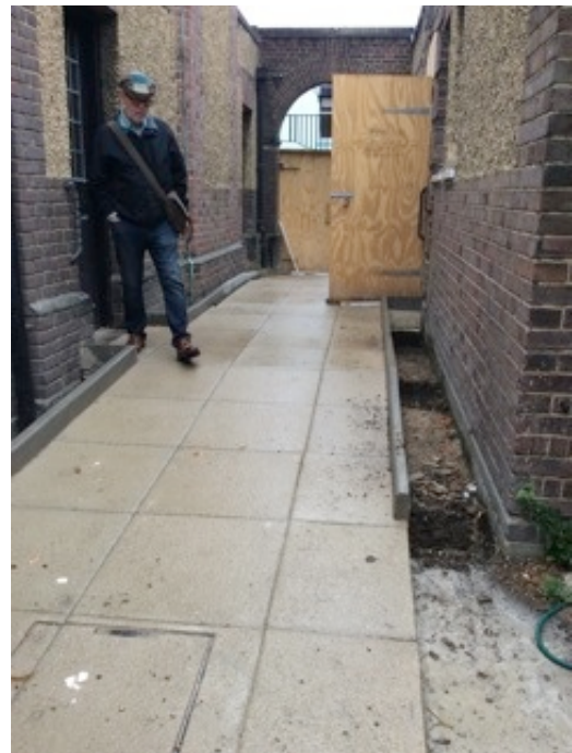
Accessibility Project. The new ramp almost complete - photographed on 29 August. Building work is expected to be finished by Friday 8 September. Official opening on 1 October.
